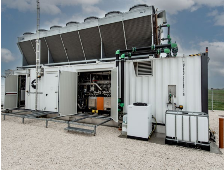
2 MW water electrolysis in Rubensdorf
